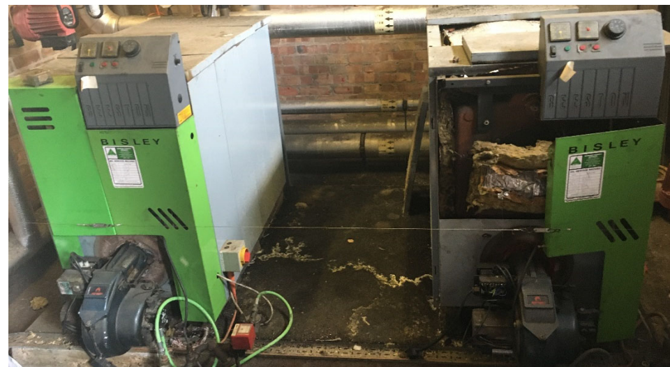
Current oil fired boilers
