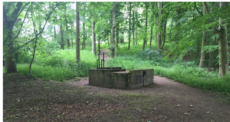
Existing foul water drainage pump
